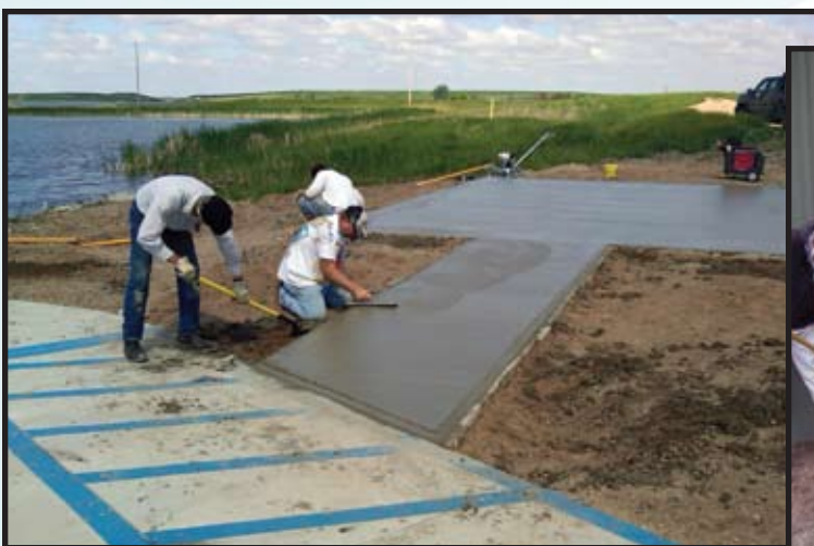
Garrison Diversion's O&M crew doing concrete work for a picnic shelter at East Park Lake.
