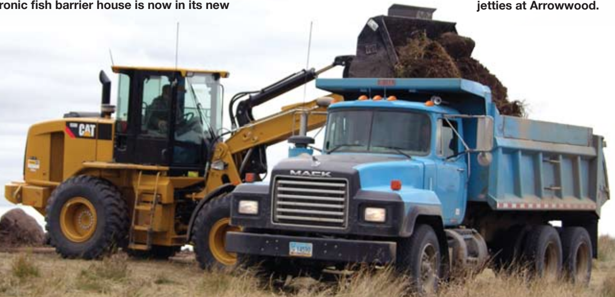
The O&M crew hauls rock to use for the jetties at Arrowwood.
