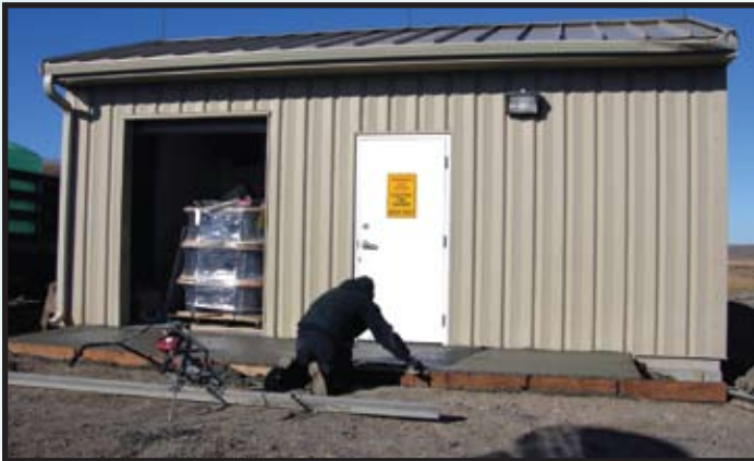
Arrowwood's electronic fish barrier house is now in its new location.
