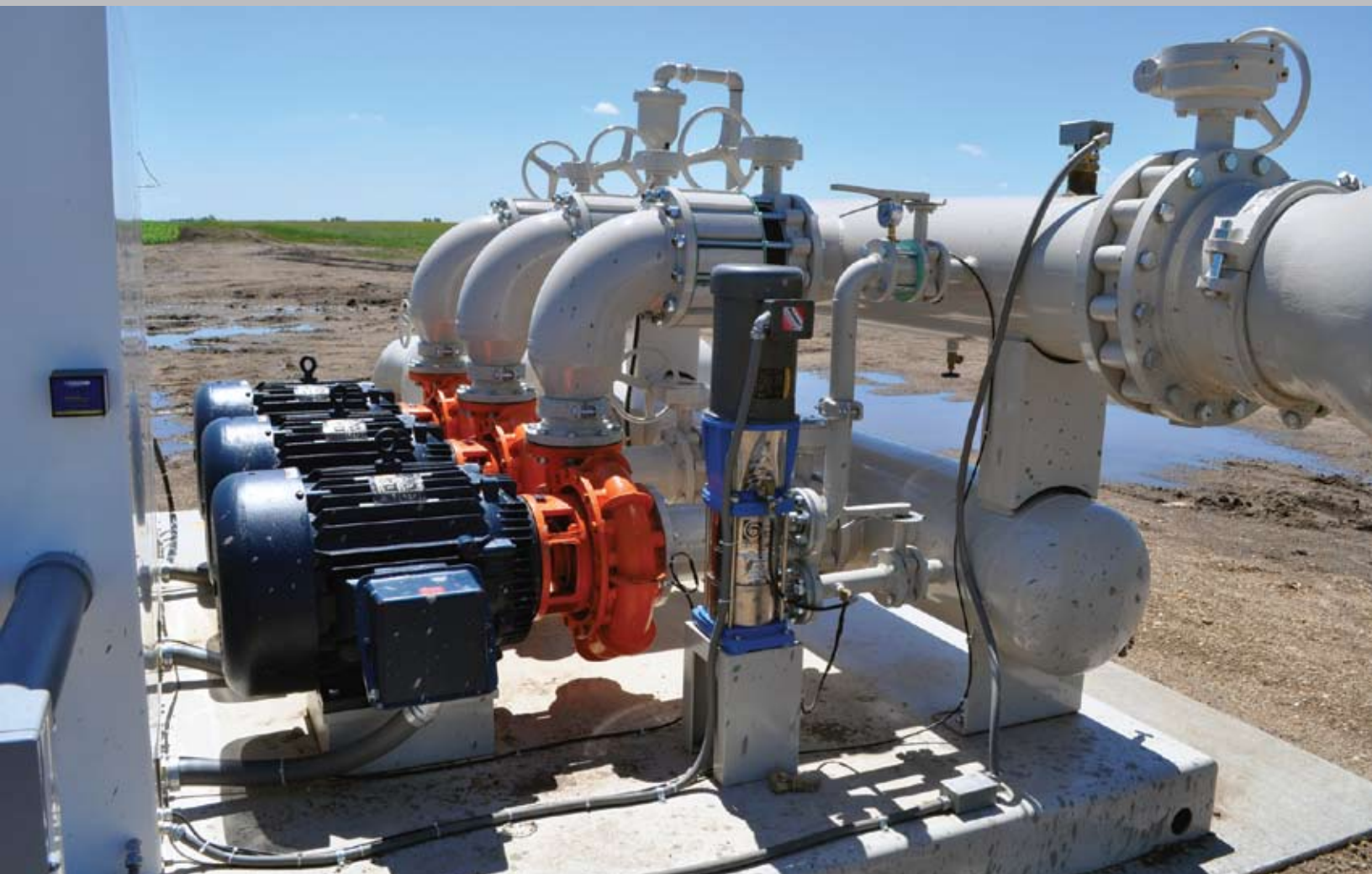
The booster station for the MM 7.5 Irrigation Project.
