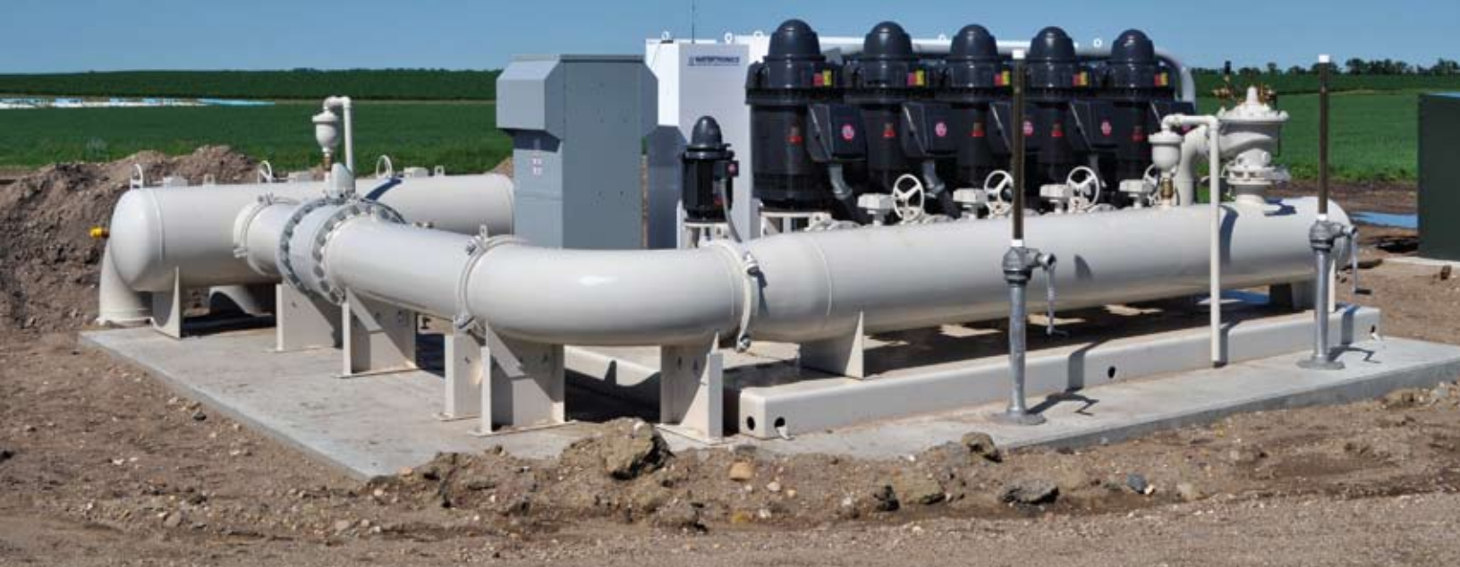
The pump station for the Mile Marker 7.5 Irrigation Project near Turtle Lake.
